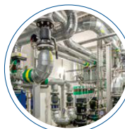
Fan and Water pump
